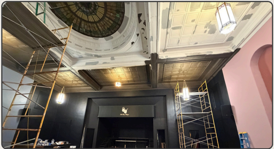
A sneak peek of the auditorium ceiling and walls as the transformation begins. Photo credit: Bryan Bible
